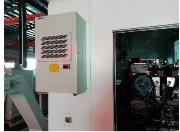
AC Cooling System
